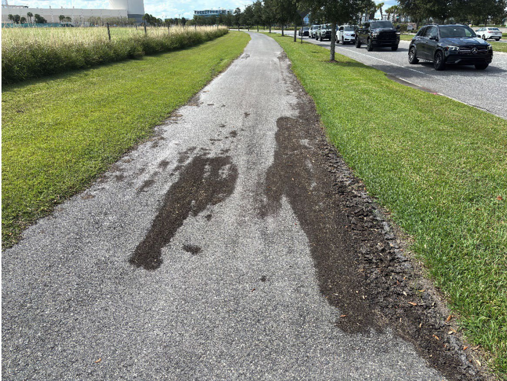
Photo 21 – Low Area Holding Water
