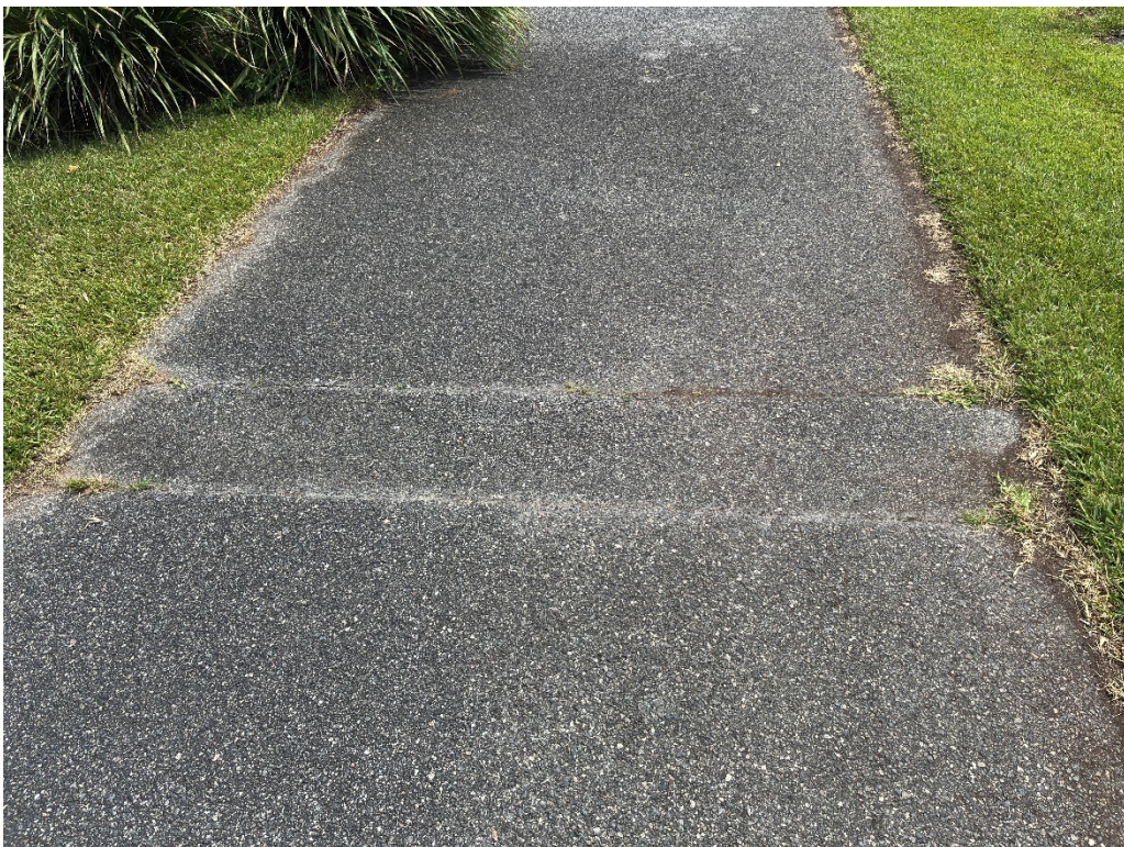
Photo 10 – Poor Quality Asphalt Patch
