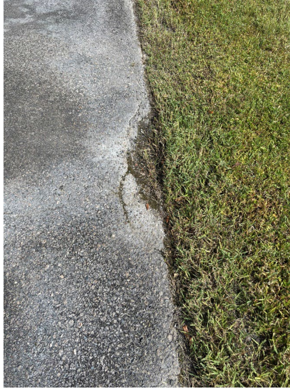
Photo 17 – Asphalt Raveling and Base Failure
