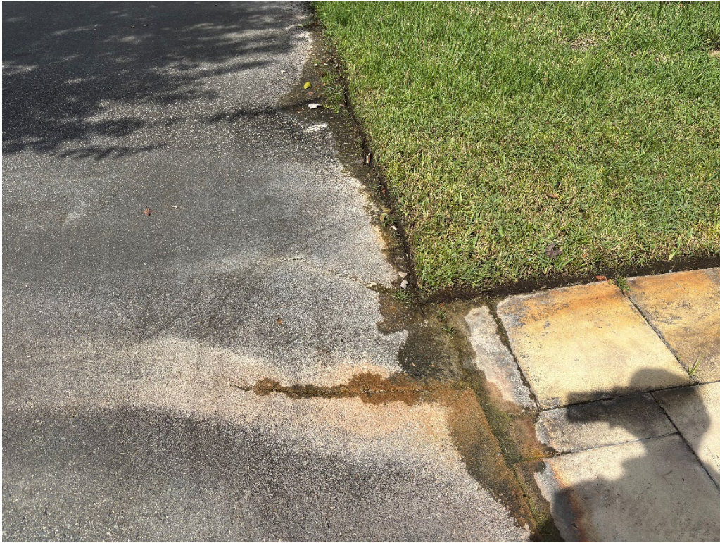
Photo 25 – Low Area Holding Water
