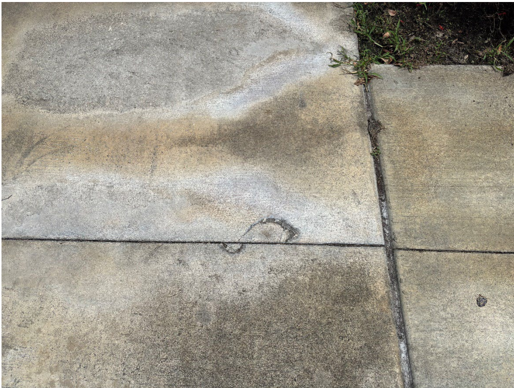
Photo 14 – Surficial Cracked Concrete
