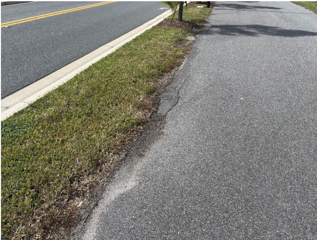
Photo 24- Asphalt Raveling and Base Failure
