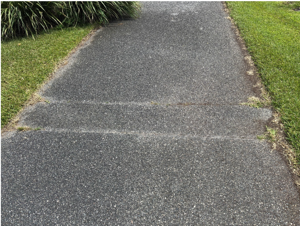
Photo 10 – Poor Quality Asphalt Patch
