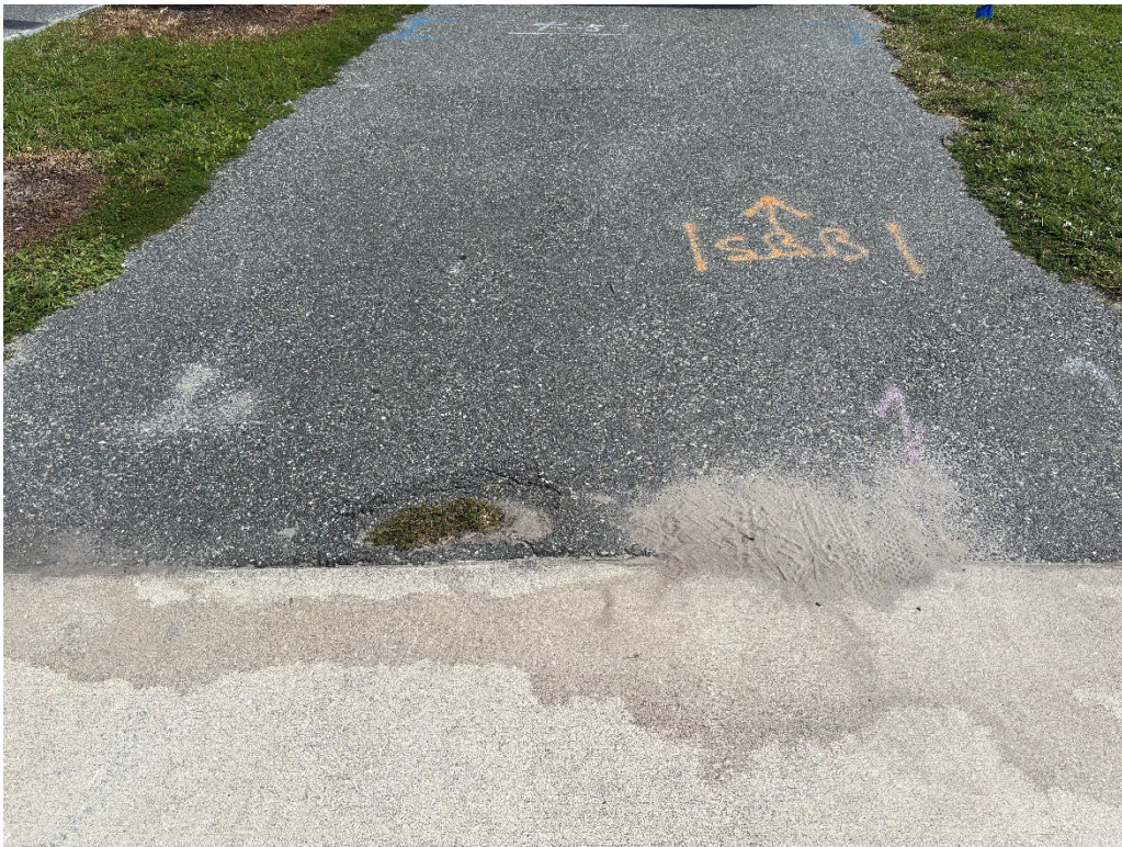
Photo 22 – Asphalt Raveling and Base Failure
