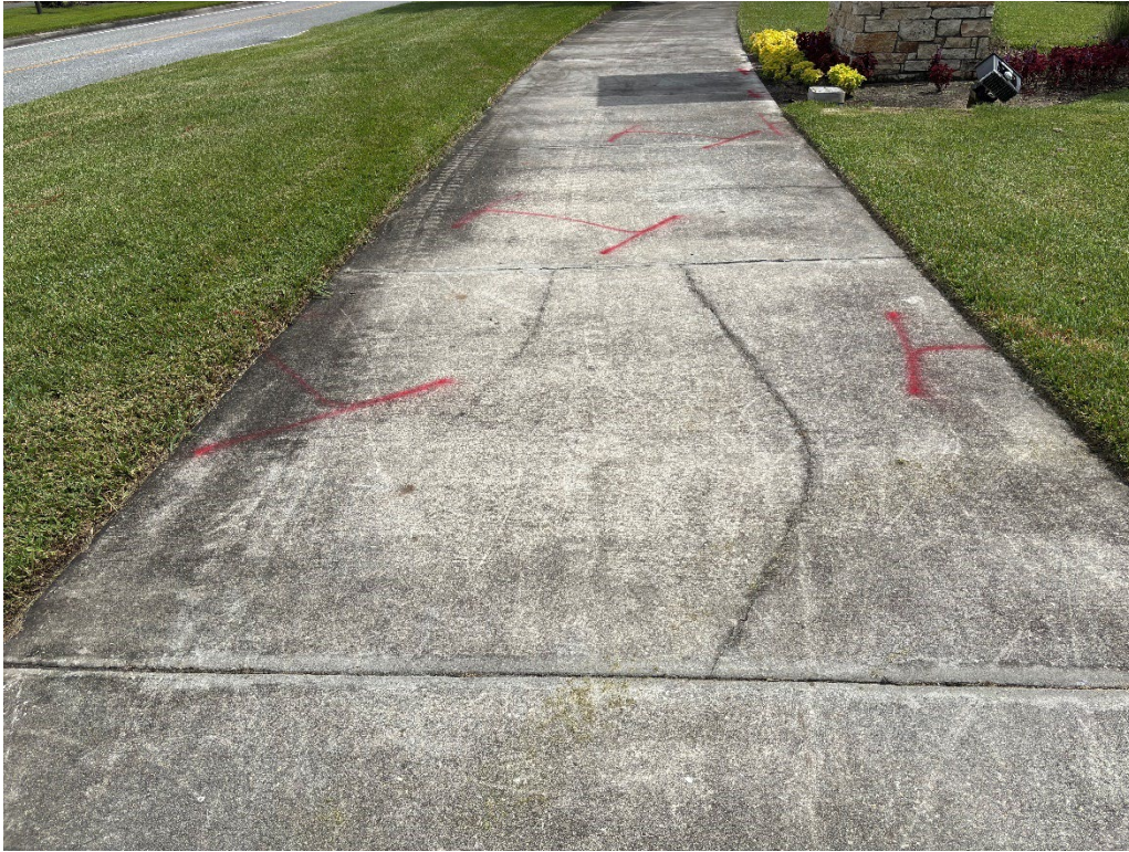
Photo 11 – Surficial Cracked Concrete
