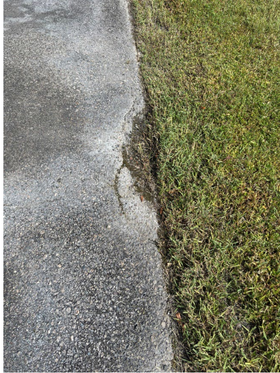
Photo 17 – Asphalt Raveling and Base Failure
