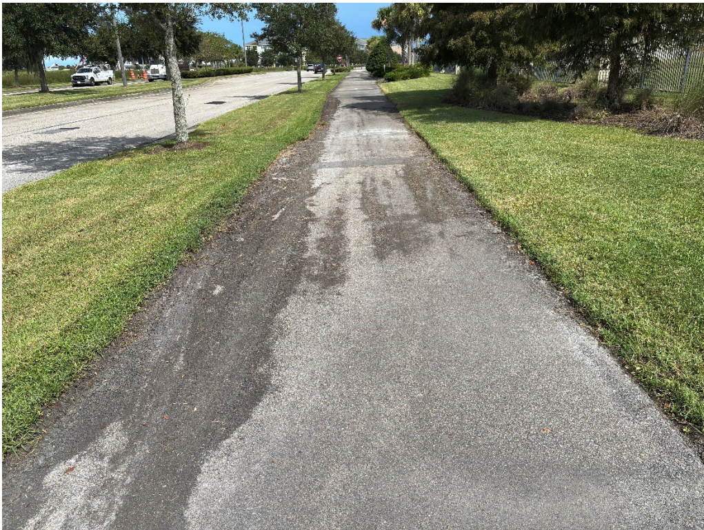
Photo 18 – Low Area Holding Water
