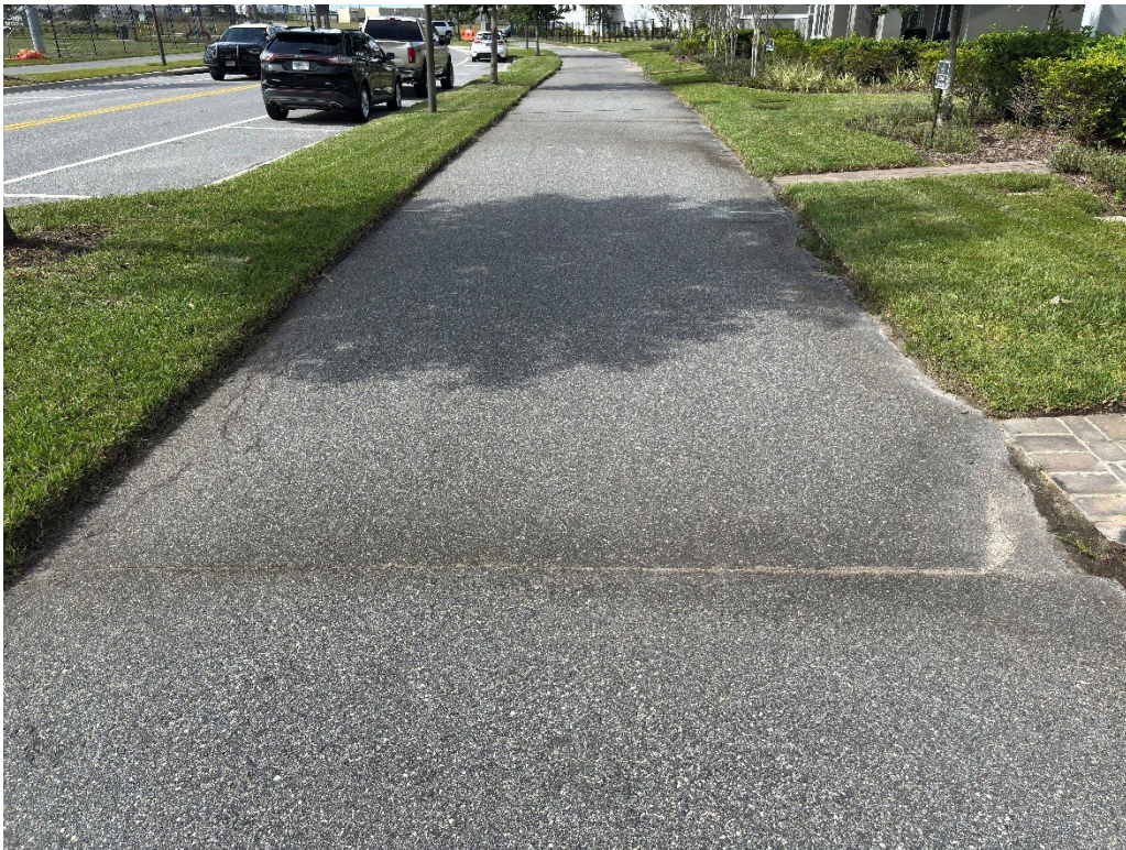
Photo 28 – Low Area Holding Water
