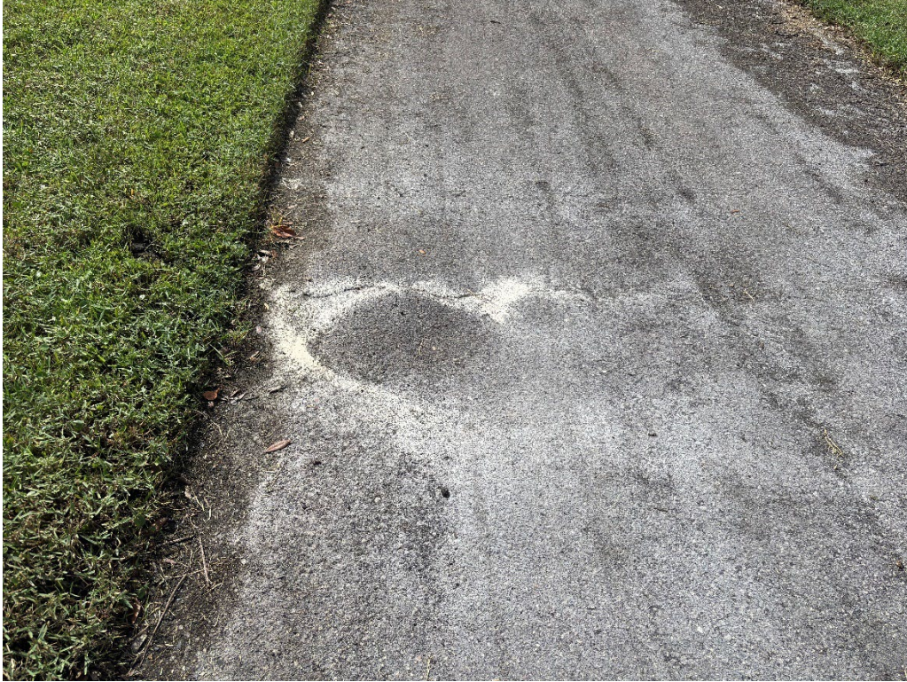
Photo 19 – Asphalt Base Failure
