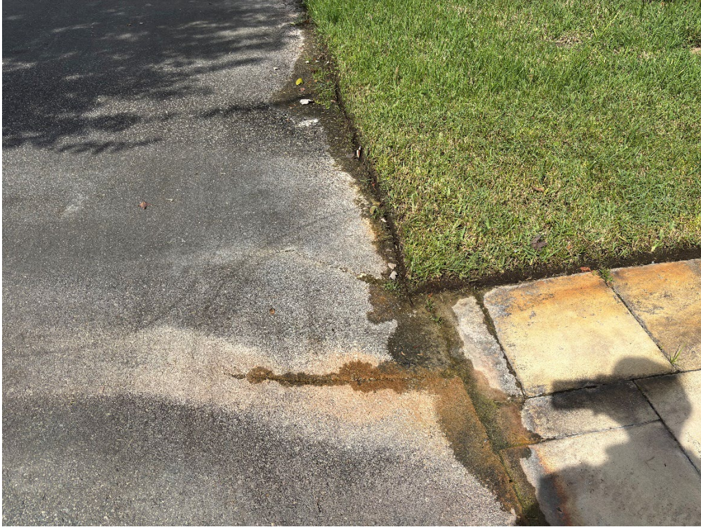
Photo 25 – Low Area Holding Water
