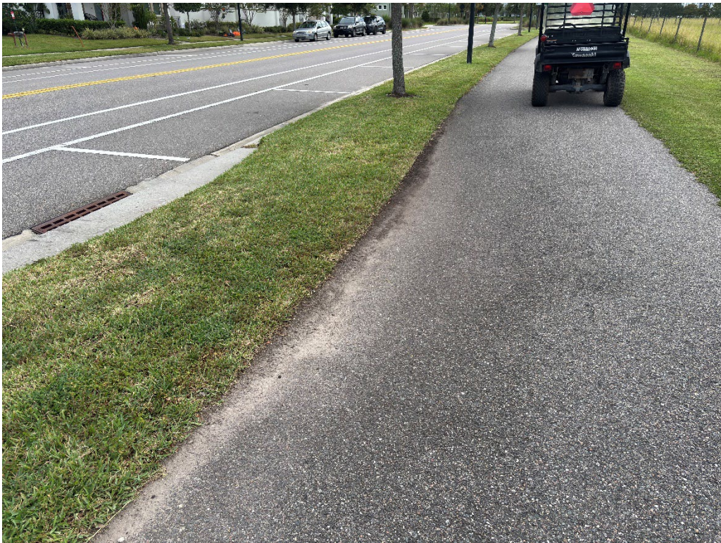
Photo 6 – Low Area Holding Water
