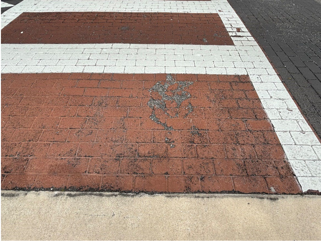
Photo 9 – Deteriorating Thermoplastic and Worn Coloration
