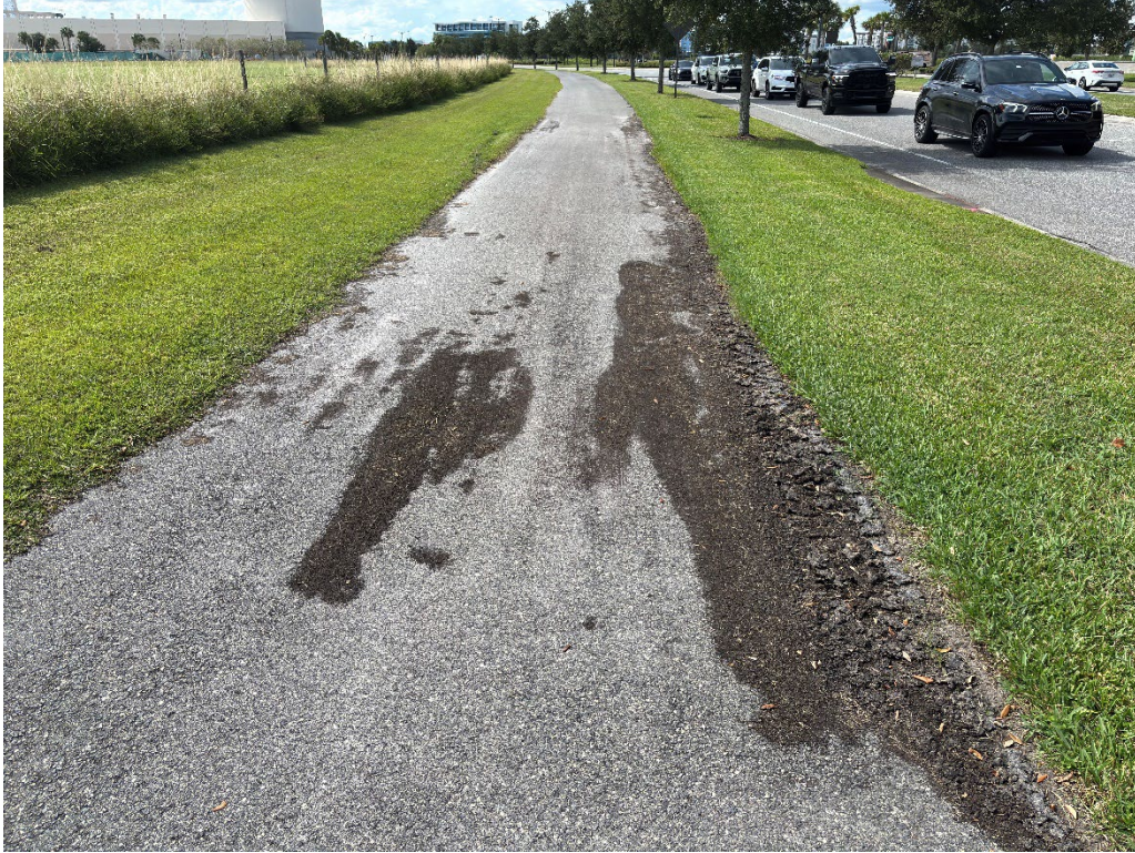
Photo 21 – Low Area Holding Water
