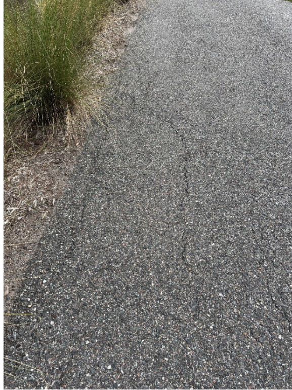
Photo 3 – Asphalt Edge Raveling
