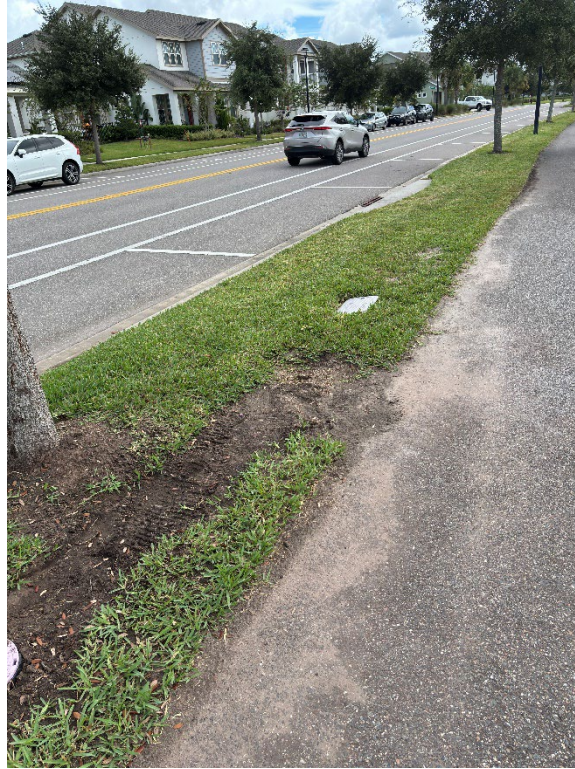
Photo 7 – Low Area Holding Water
