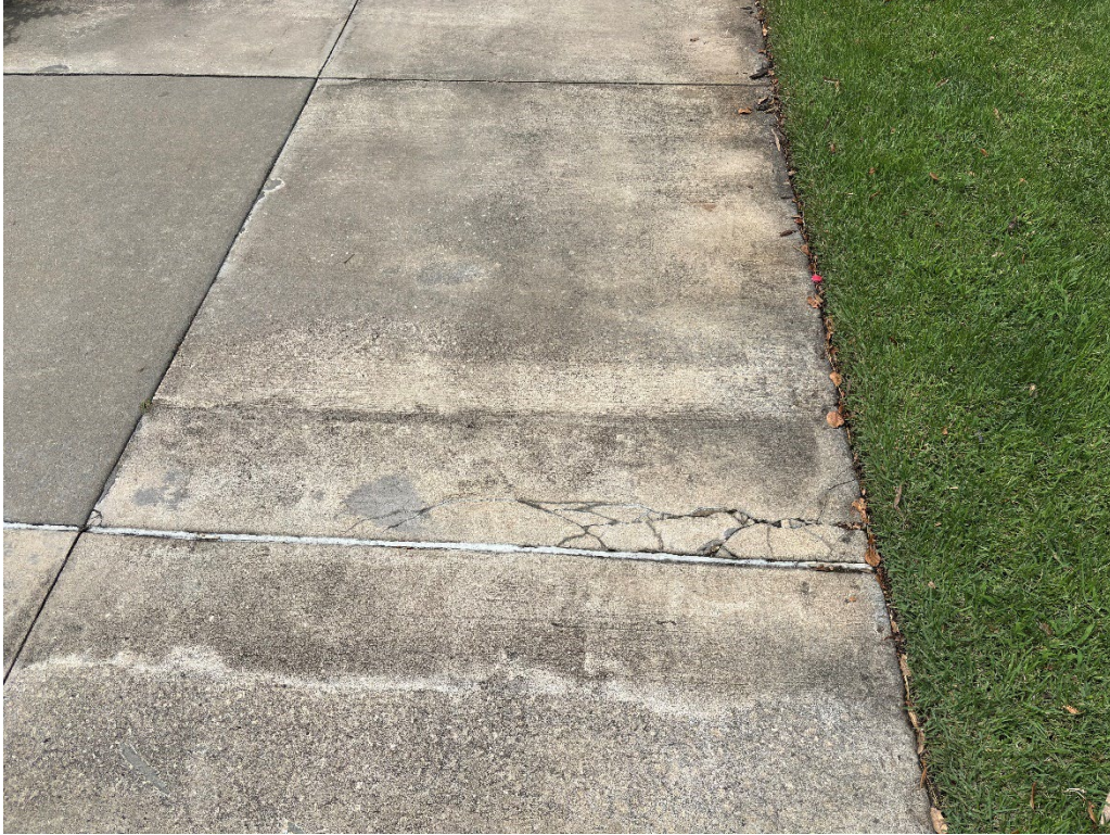
Photo 13 – Surficial Cracked Concrete
