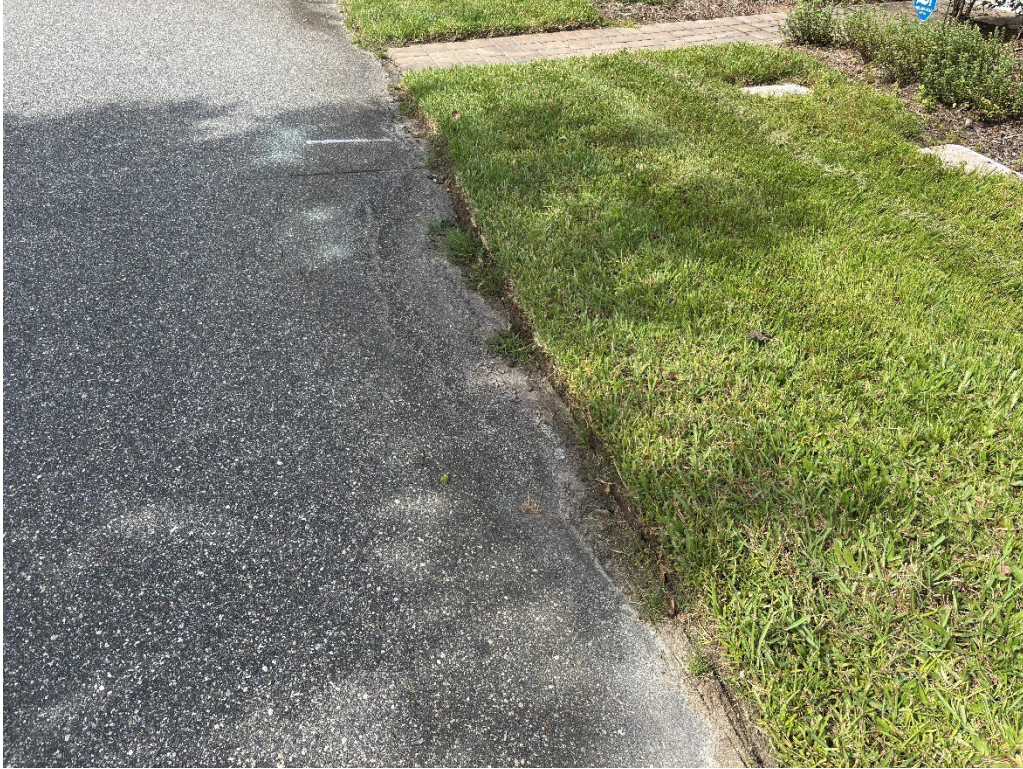
Photo 29 – Asphalt Raveling and Base Failure
