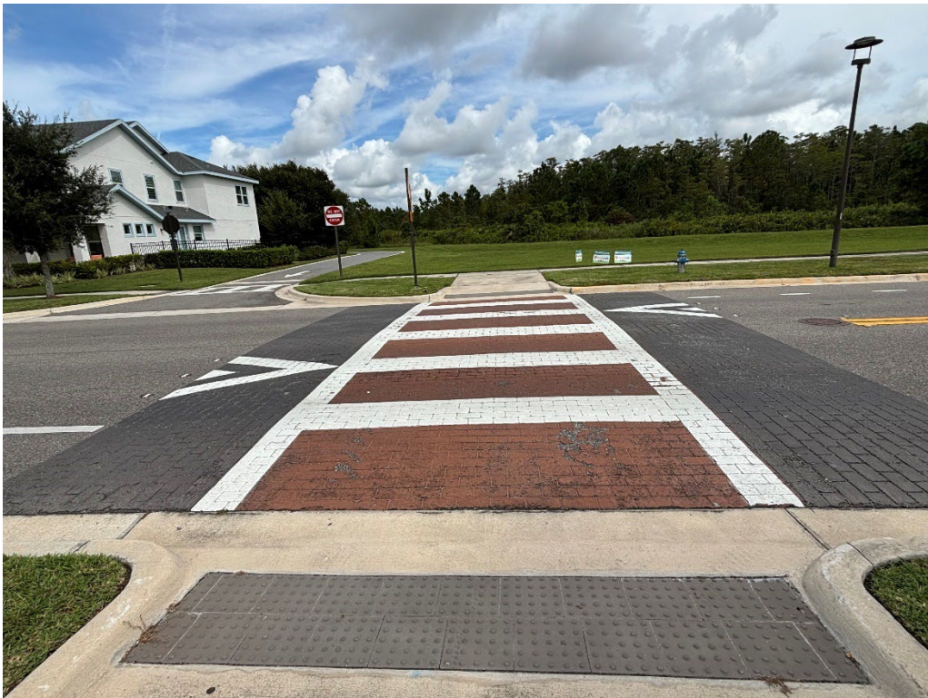
Photo 8 – Deteriorating Thermoplastic and Worn Coloration
