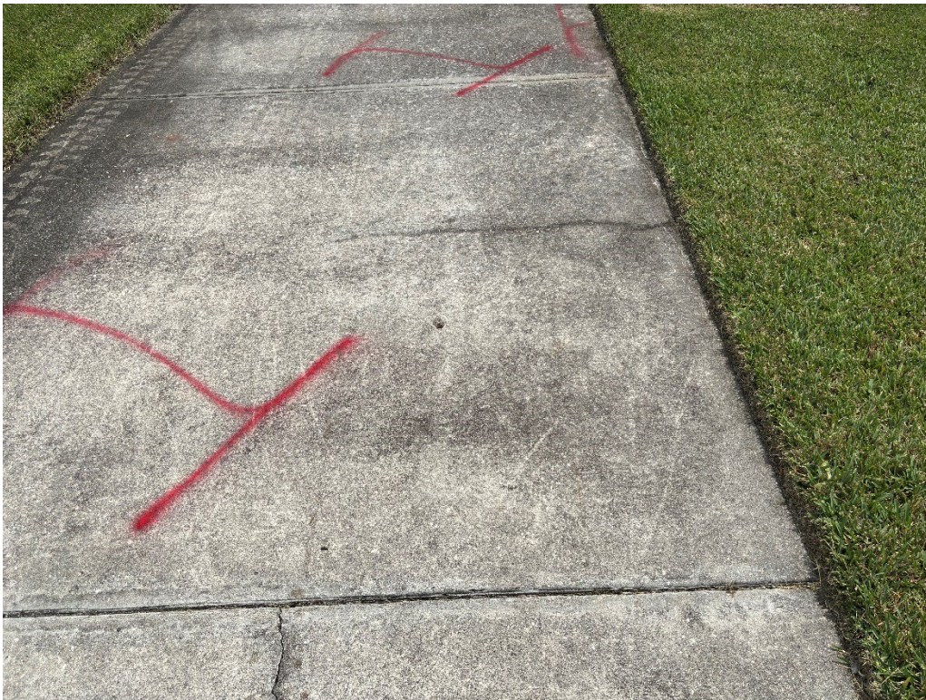
Photo 12 – Surficial Cracked Concrete
