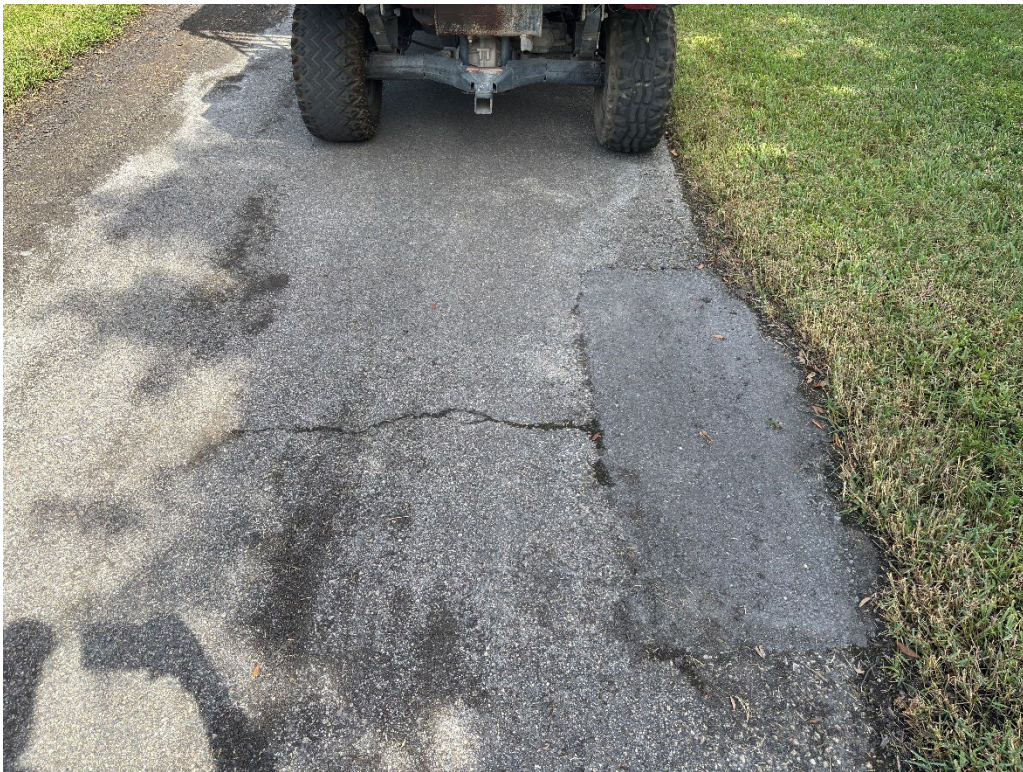
Photo 20 – Poor Quality Asphalt Patch
