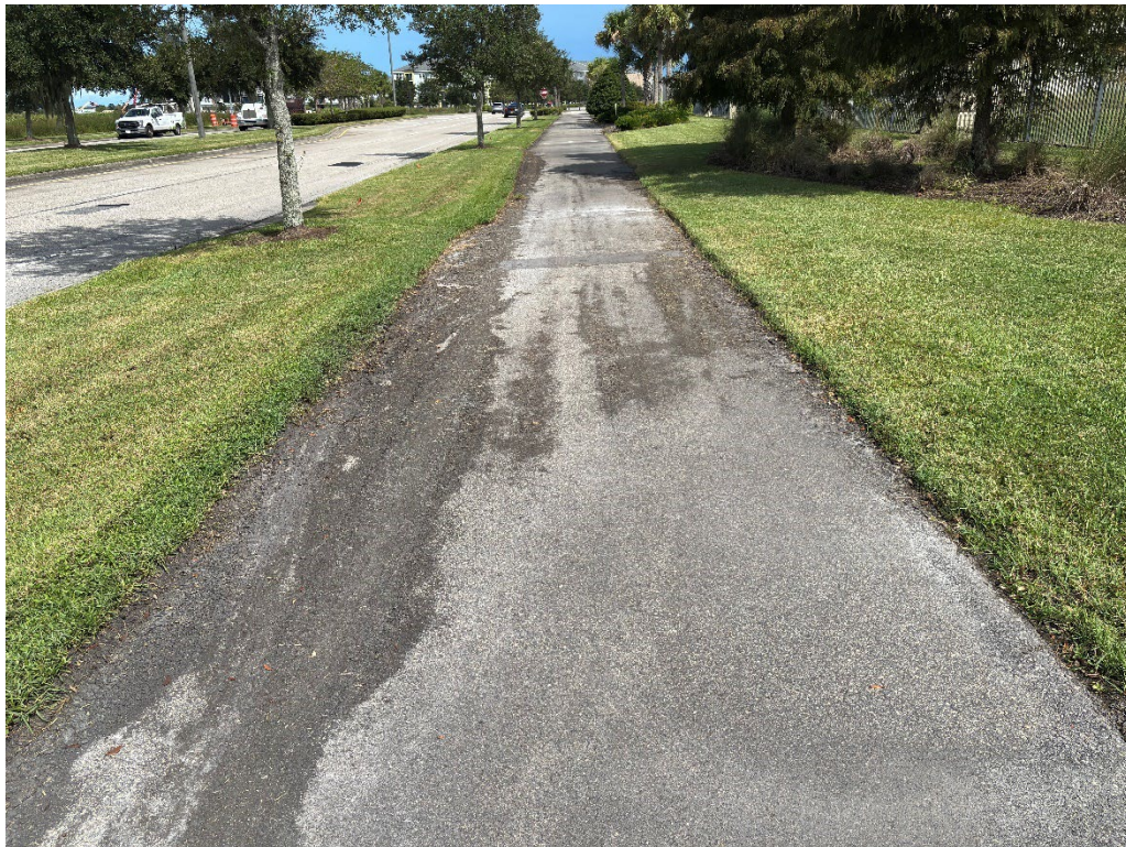
Photo 18 – Low Area Holding Water
