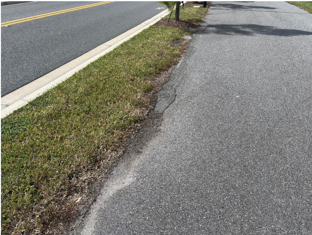
Photo 24- Asphalt Raveling and Base Failure
