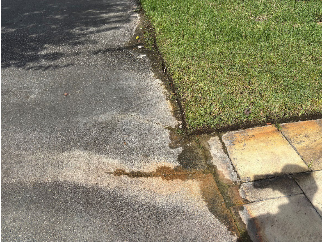
Photo 25 – Low Area Holding Water
