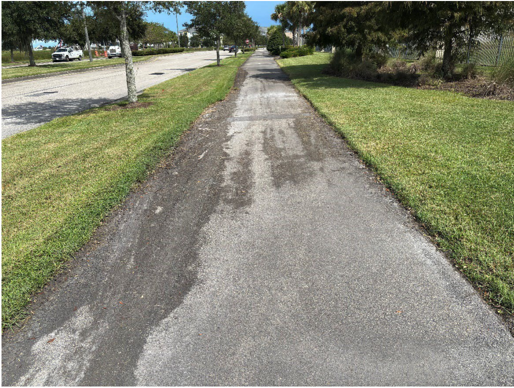
Photo 18 – Low Area Holding Water
