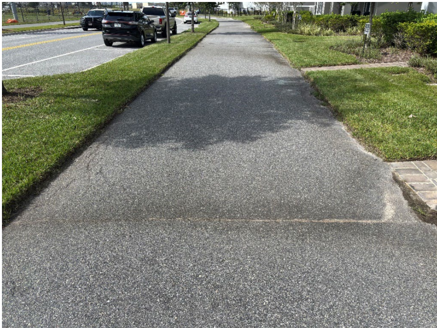
Photo 21 - Cracked Asphalt from Side to Side (No Observed Changes) (Refer to Prior Photo 28 – 2025 Assessment)
