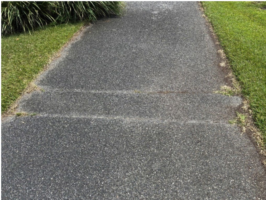
Photo 10 - Cracked Asphalt from Side to Side (No Observed Changes) (Refer to Prior Photo 10 – 2025 Assessment)
