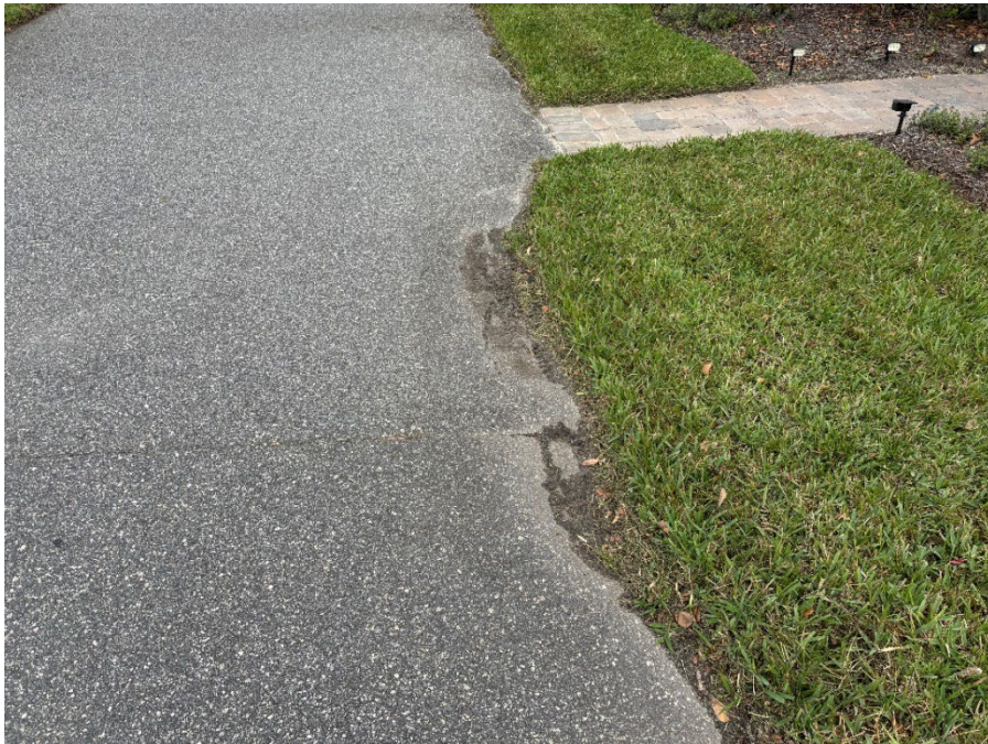
Photo 22 - Asphalt Raveling and Base Failure (No Observed Changes) (Refer to Prior Photo 29 – 2025 Assessment)
