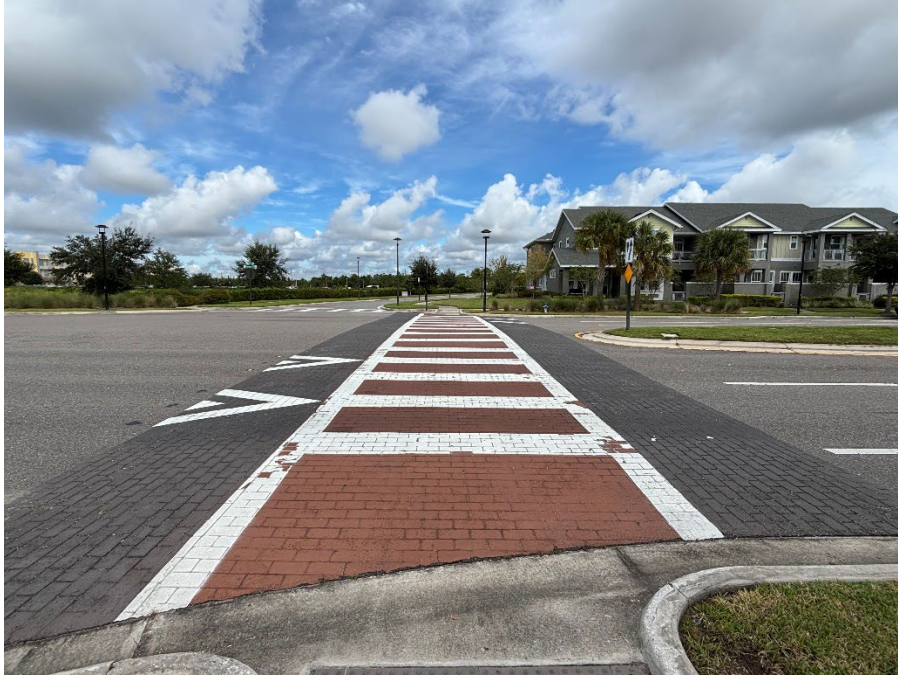
Photo 1 Deteriorating Thermoplastic and Worn Coloration (No Observed Changes) (Refer to Prior Photo 1 – 2025 Assessment)
