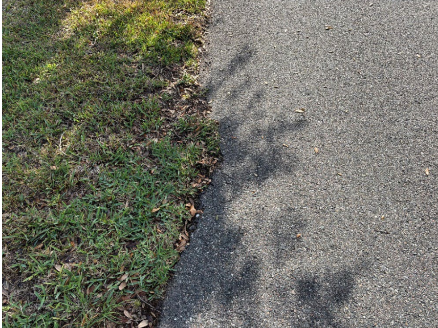
Photo 7.1 – Asphalt Edge Failure (New Photo – 2026 Assessment)
