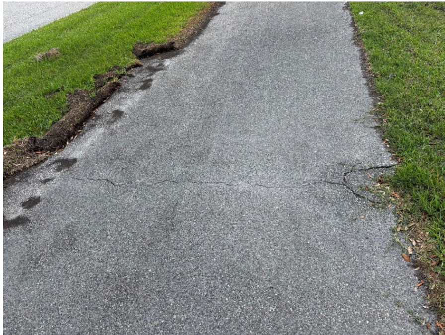
Photo 18.1 - Asphalt Raveling and Base Failure, Cracked Asphalt from Side to Side (New Photo – 2026 Assessment)
