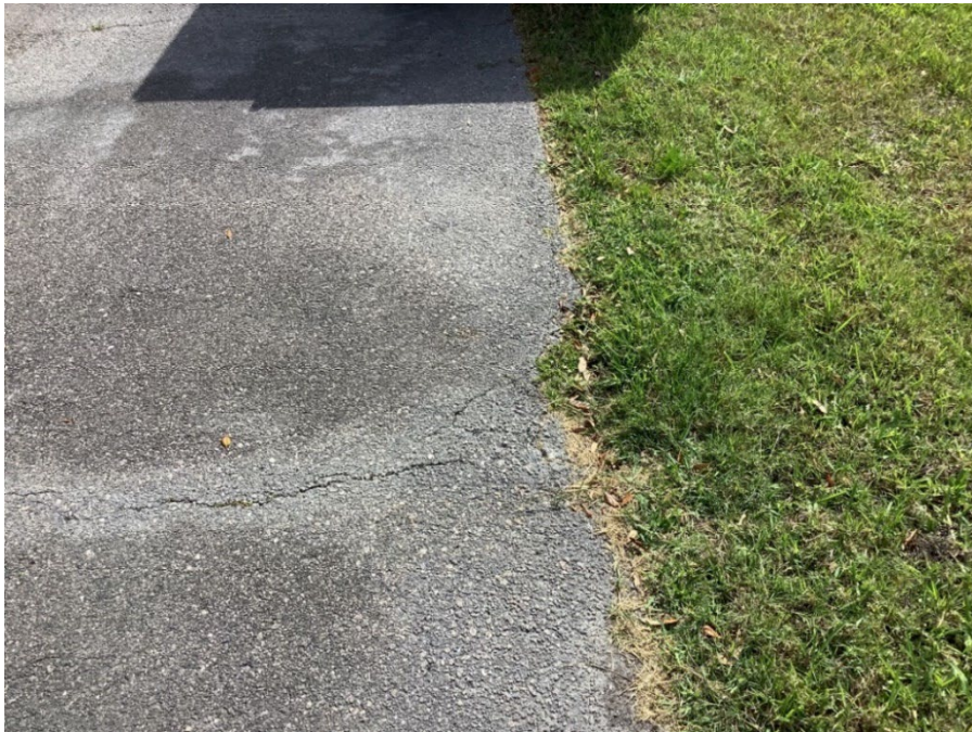
Photo 16 - Asphalt Raveling and Base Failure (Further Edge Failure Observed and Cracked Asphalt from Side to Side) (Refer to Prior Photo 17 – 2025 Assessment)
