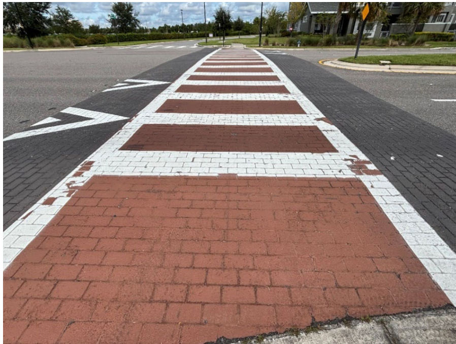
Photo 2 Deteriorating Thermoplastic and Worn Coloration (No Observed Changes) (Refer to Prior Photo 2 – 2025 Assessment)
