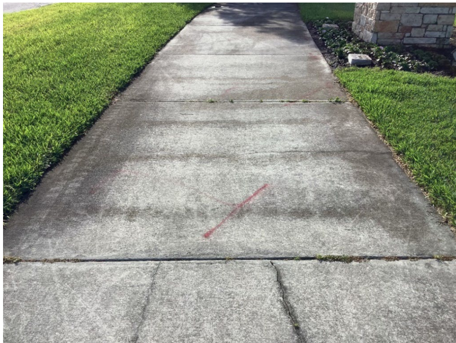
Photo 12 - Surficial Cracked Concrete (No Observed Changes) (Refer to Prior Photo 12 – 2025 Assessment)
