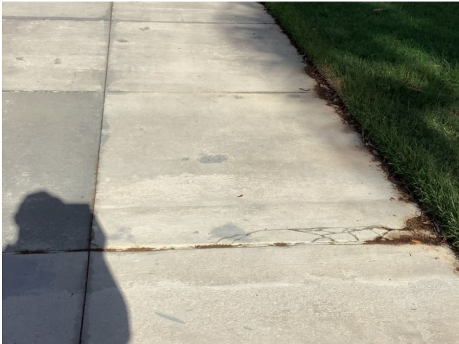
Photo 13 - Cracked Concrete (No Observed Changes) (Refer to Prior Photo 13 – 2025 Assessment)
