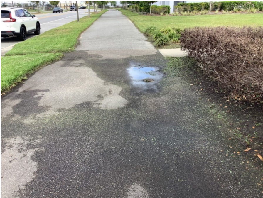
Photo 19.1 - Low Area Holding Water, Asphalt Raveling and Base Failure (New Photo – 2026 Assessment)
