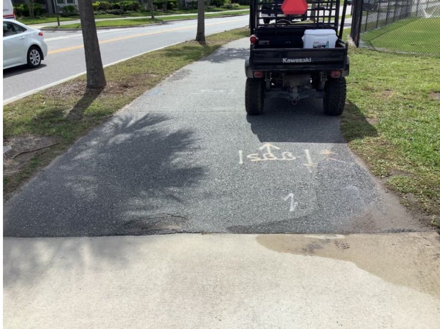
Photo 18 - Asphalt Raveling and Base Failure (No Observed Changes) (Refer to Prior Photo 22 – 2025 Assessment)
