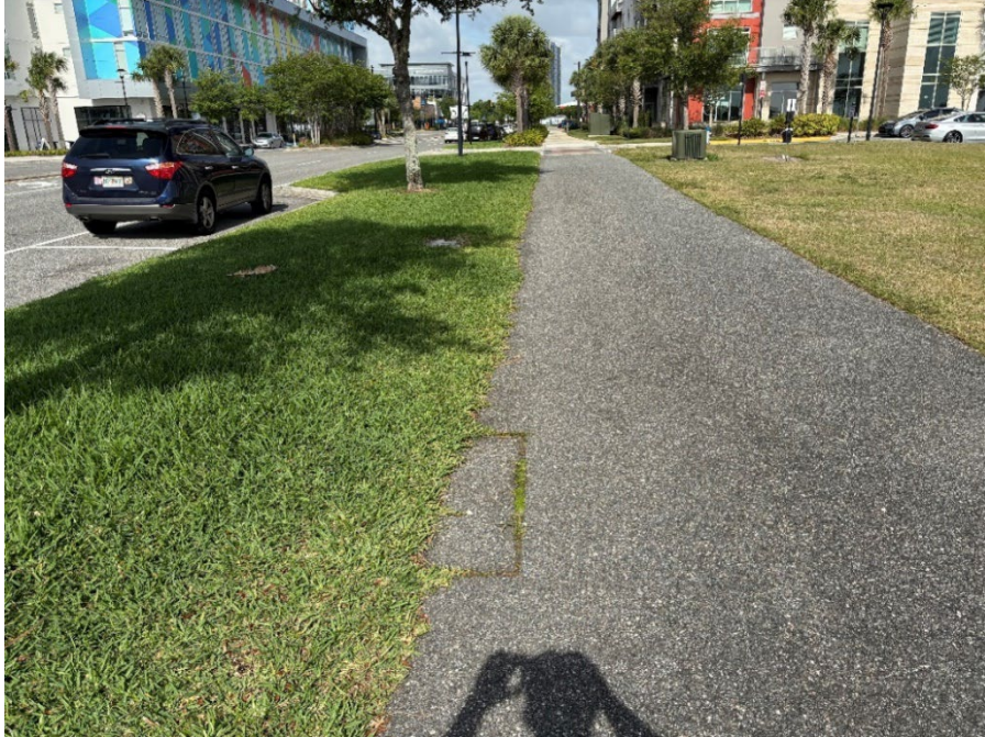
Photo 12.1 - Poor Quality Asphalt Patch (New Photo – 2026 Assessment)
