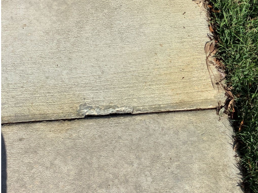
Photo 15.1 Broken Concrete (New Photo – 2026 Assessment)
