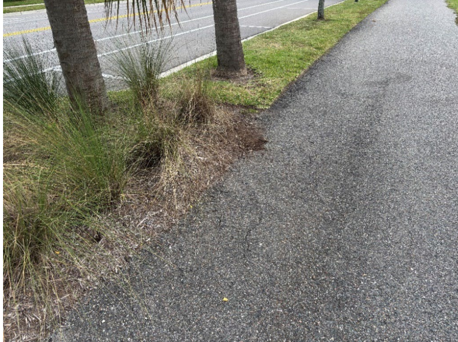
Photo 3 Asphalt Edge Raveling (Increased Asphalt Raveling Observed) (Refer to Prior Photo 3 – 2025 Assessment)
