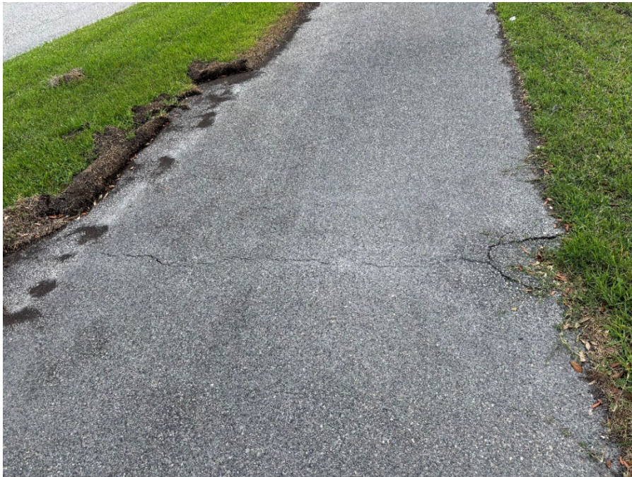
Photo 18.1 - Asphalt Raveling and Base Failure, Cracked Asphalt from Side to Side (New Photo – 2026 Assessment)
