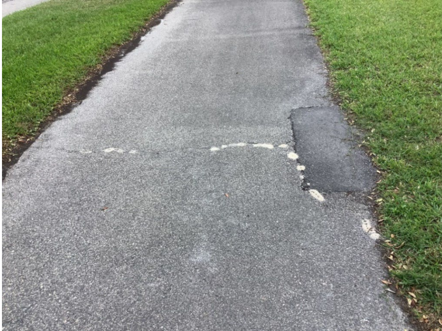
Photo 17 - Poor Quality Asphalt Patch (No Observed Changes) (Refer to Prior Photo 20 – 2025 Assessment)
