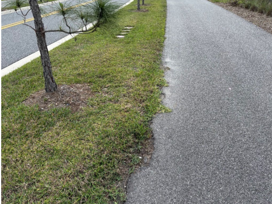
Photo 21.1 - Asphalt Edge Failure (New Photo – 2026 Assessment)
