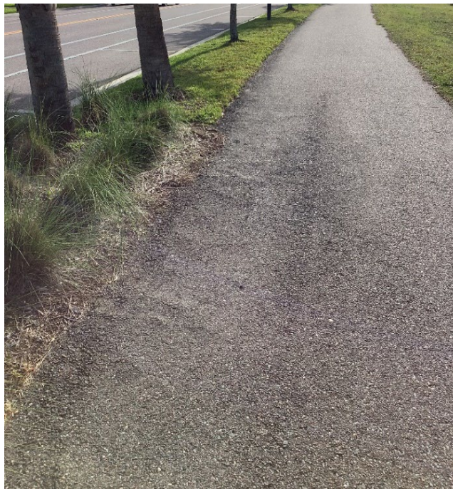
Photo 5 - Asphalt Raveling (Increased Asphalt Raveling Observed) (Refer to Prior Photo 5 – 2025 Assessment)
