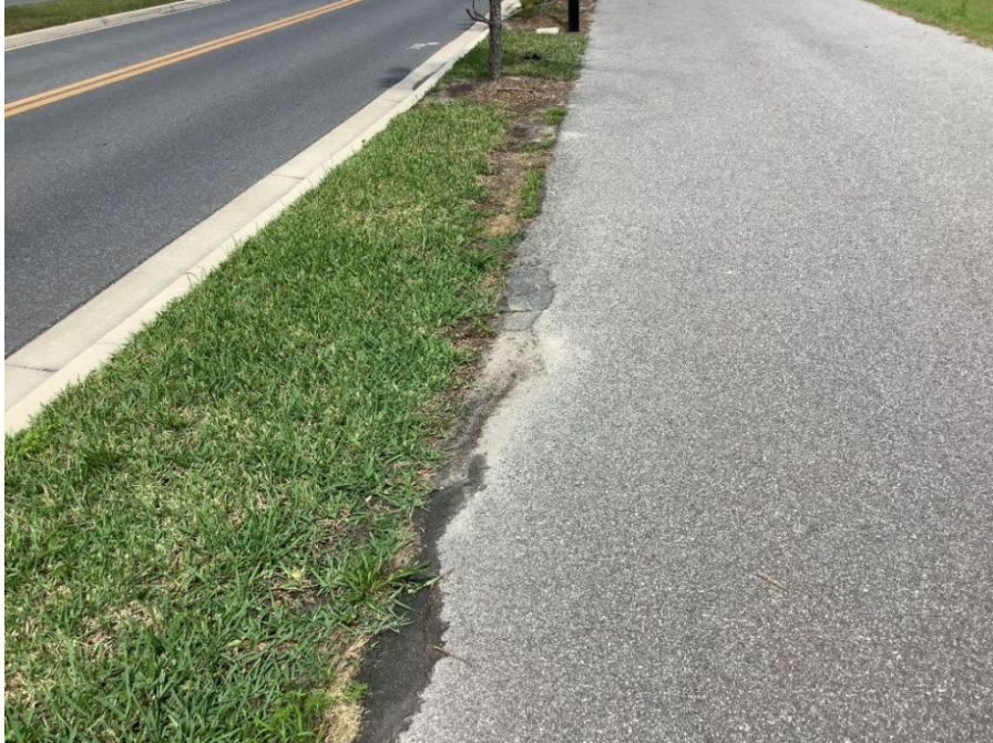
Photo 19 - Asphalt Raveling and Base Failure (No Observed Changes) (Refer to Prior Photo 24 – 2025 Assessment)
