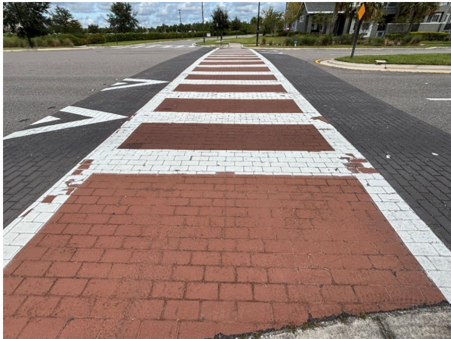
Photo 2 Deteriorating Thermoplastic and Worn Coloration (No Observed Changes) (Refer to Prior Photo 2 – 2025 Assessment)
