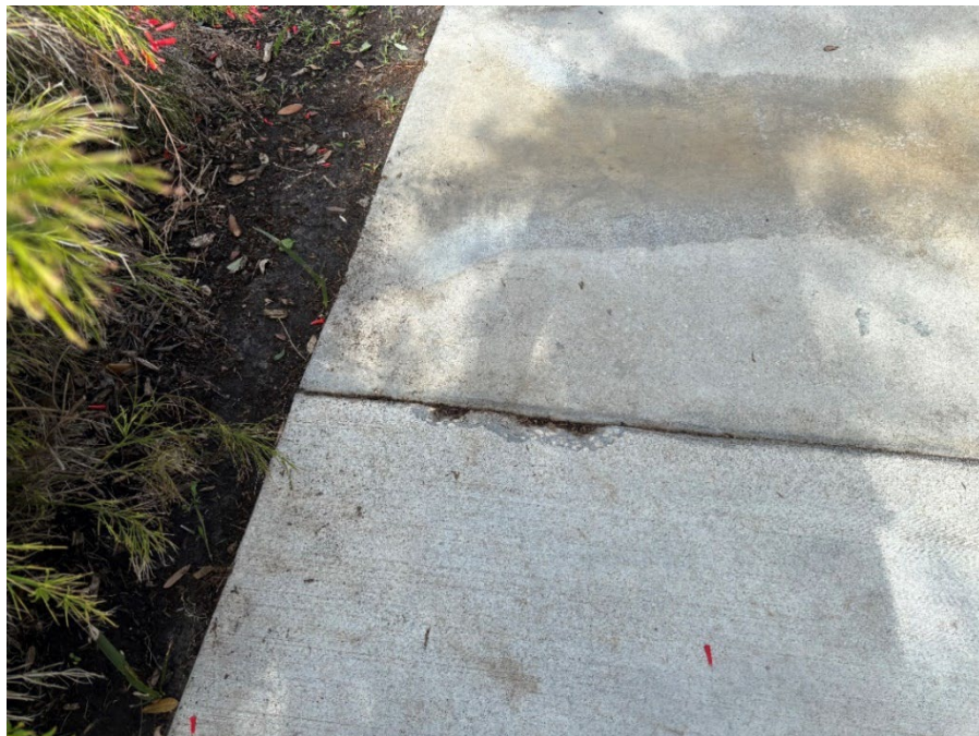
Photo 15 - Broken Concrete (No Observed Changes) (Refer to Prior Photo 15 – 2025 Assessment)
