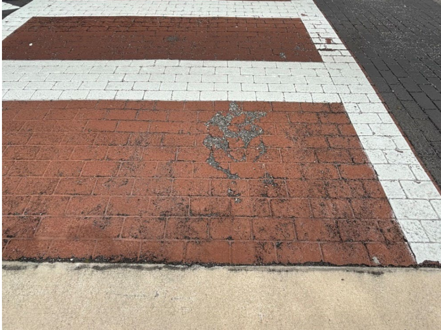
Photo 9 Deteriorating Thermoplastic and Worn Coloration (No Observed Changes) (Refer to Prior Photo 9 – 2025 Assessment)
