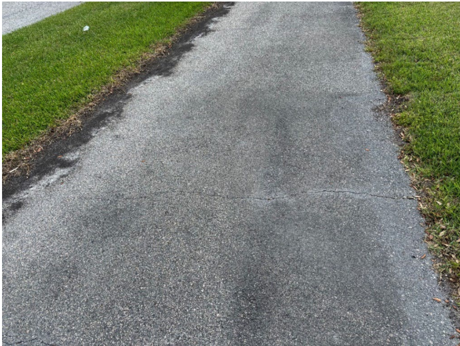
Photo 17.1 - Cracked Asphalt from Side to Side (New Photo – 2026 Assessment)
