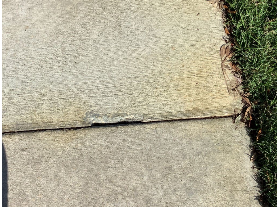
Photo 15.1 Broken Concrete (New Photo – 2026 Assessment)
