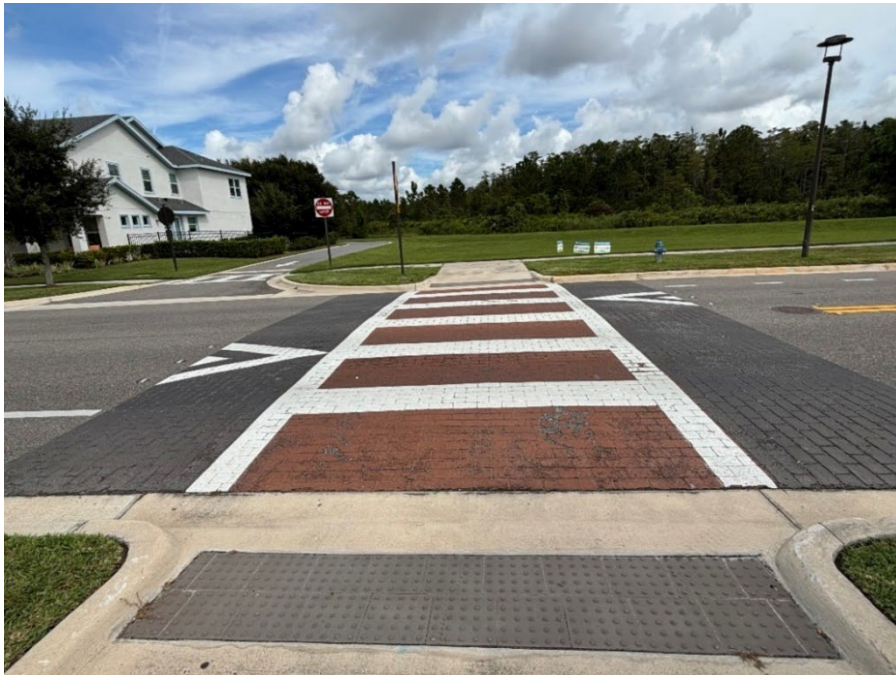
Photo 8 Deteriorating Thermoplastic and Worn Coloration (No Observed Changes) (Refer to Prior Photo 8 – 2025 Assessment)
