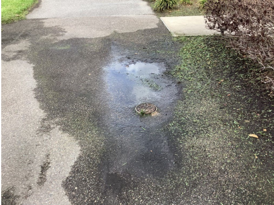
Photo 20 – Valve Cover Reveal ½ -inch (Low Area Holding Water, Asphalt Raveling and Base Failure) (Refer to Prior Photo 26 – 2025 Assessment)
