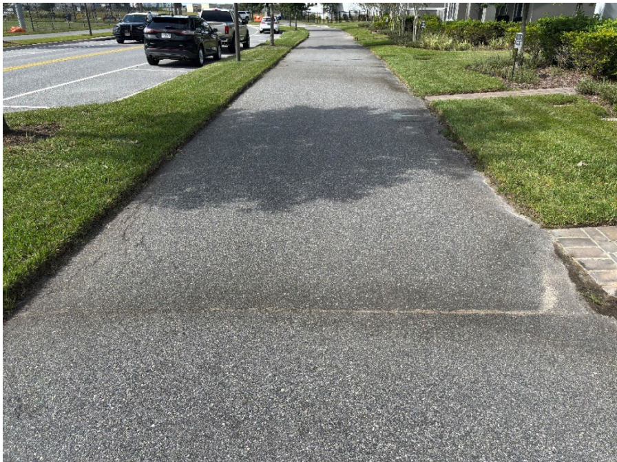
Photo 21 - Cracked Asphalt from Side to Side (No Observed Changes) (Refer to Prior Photo 28 – 2025 Assessment)
